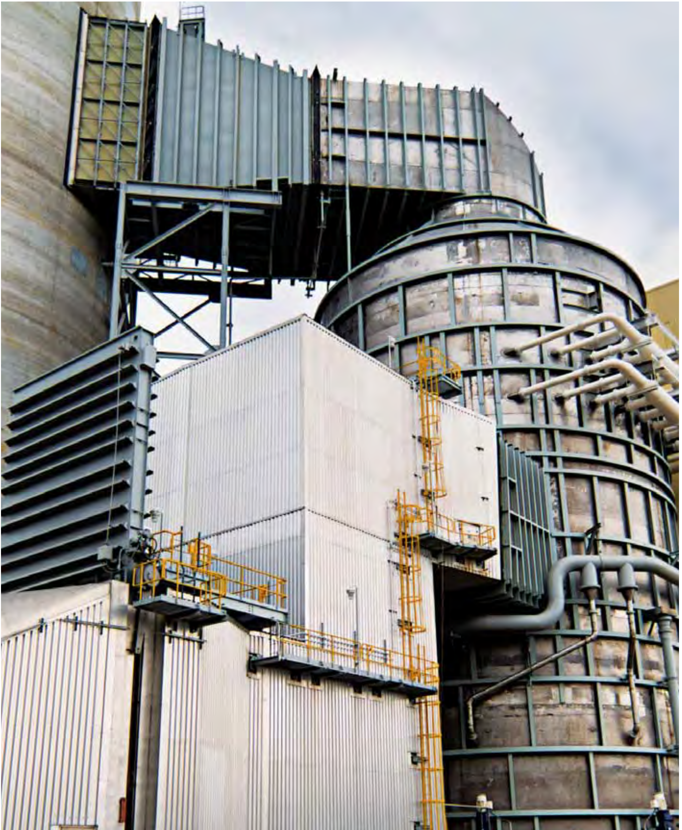
A scrubber installed at a plant
