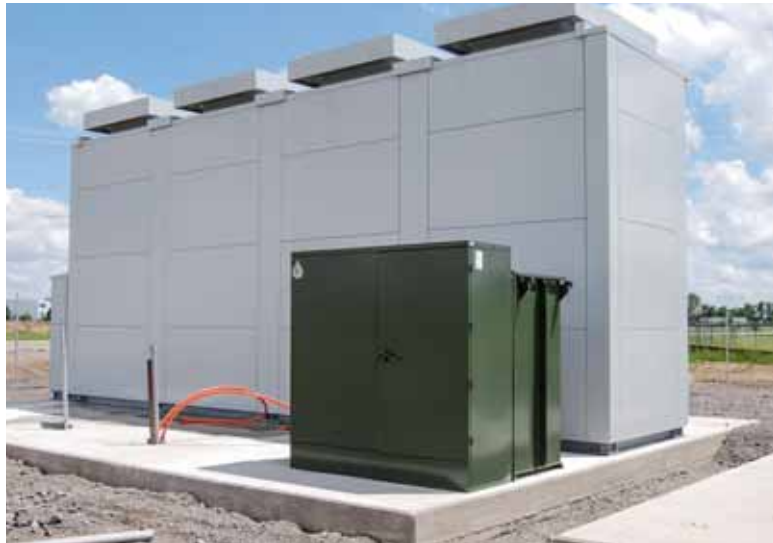
New large-capacity storage batteries are tested to support current load in several areas.
