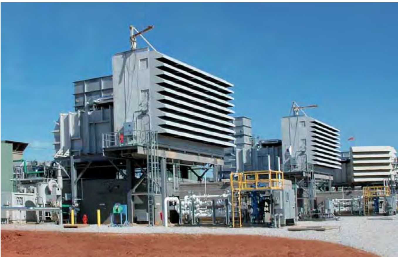
SWEPCO Mattison peaking plant
