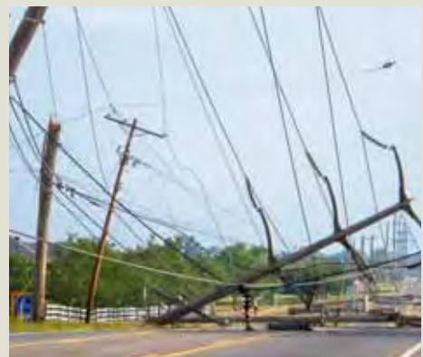
The 2012 derecho toppled hundreds of poles and lines throughout AEP’s service area.
