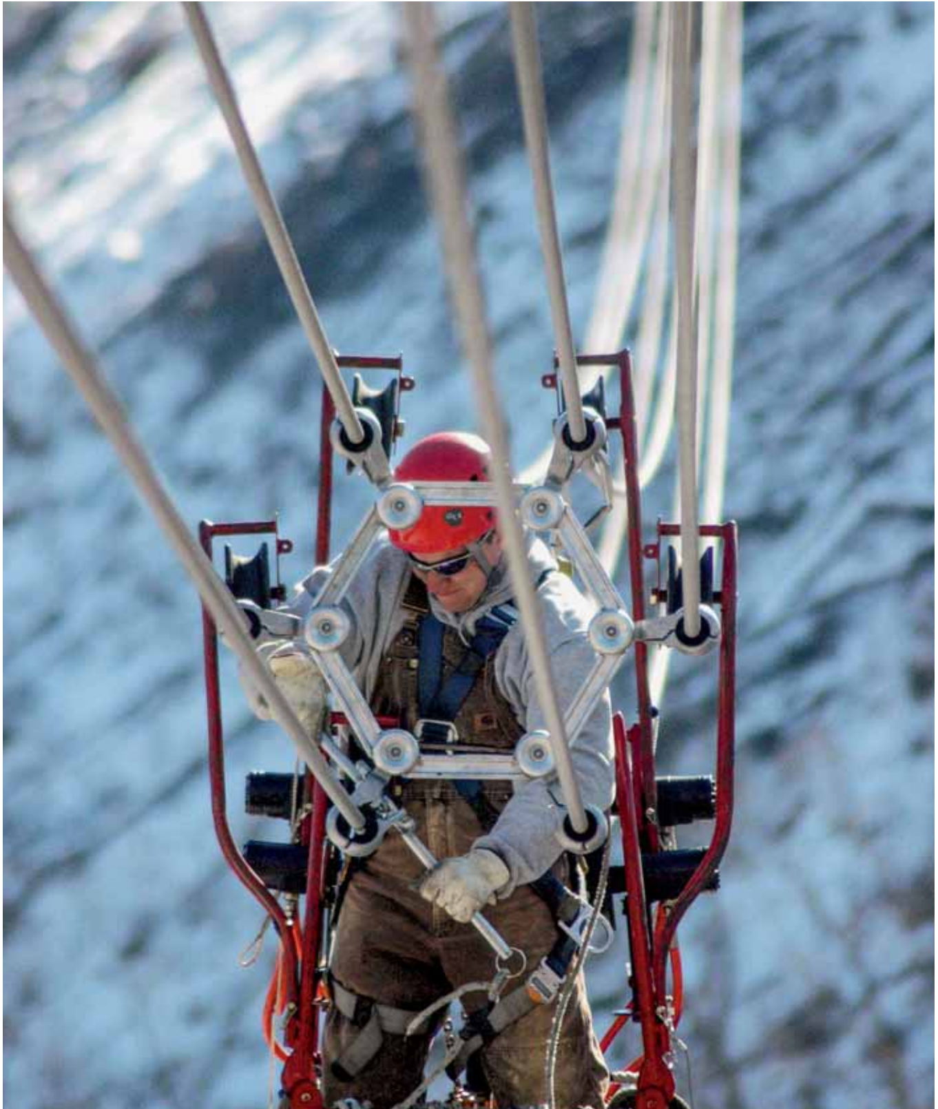
AEP's six-bundle spacers provide increased service along the Wyoming-Jackson Ferry Line in West Virginia.
