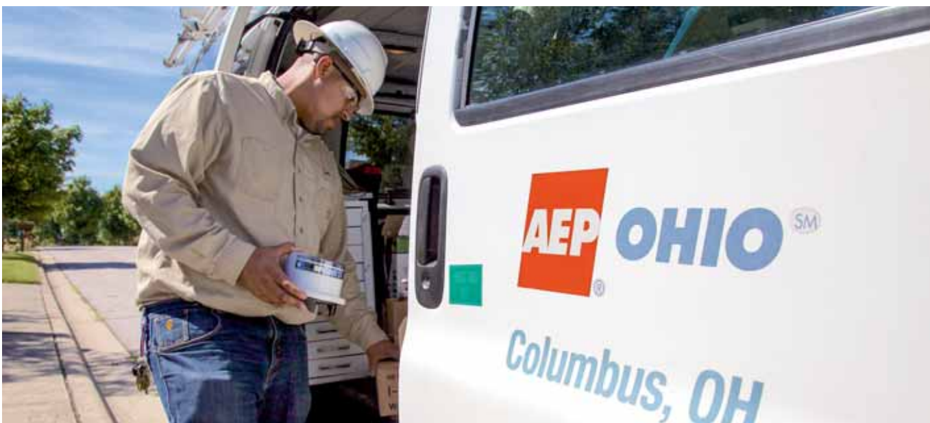
An AEP Ohio employee prepares to install a smart meter in central Ohio as part of the gridSMART demonstration project.
