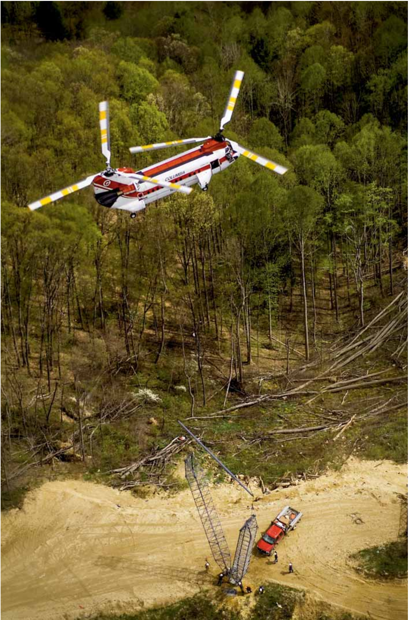
Construction on AEP's network of 765-kilovolt lines, the largest in the nation
