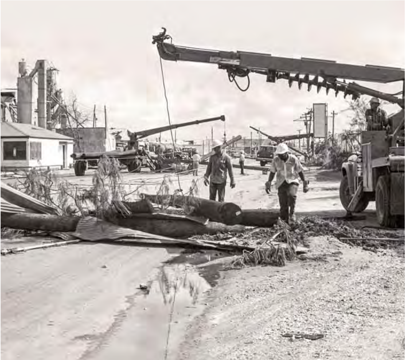
Employees of Central Power and Light and other utilities worked around the clock after Hurricane Celia to return service to normal.
