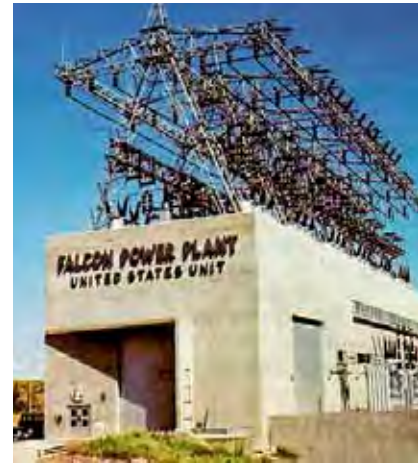
The United States Unit of the Falcon Power Plant generated power for both countries across international borders.
