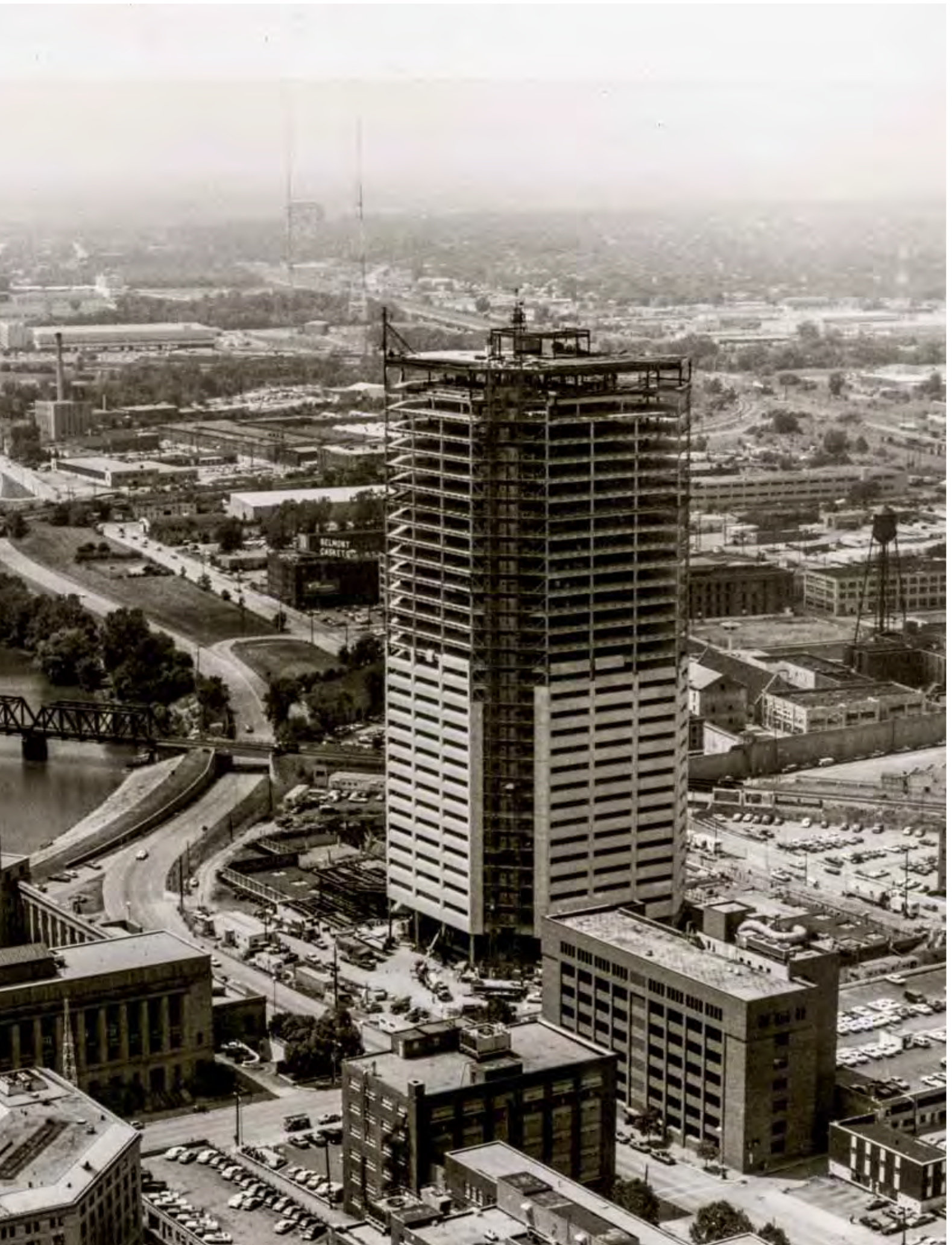
Construction of AEP's custom-built all-electric headquarters in the heart of Columbus, Ohio
