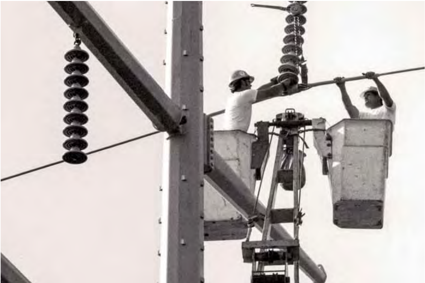
A 138,000-volt transmission line in PSO territory
