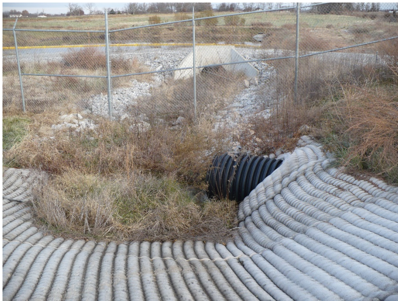
Photo #7 – sediment deposit at outlet of northeast letdown
