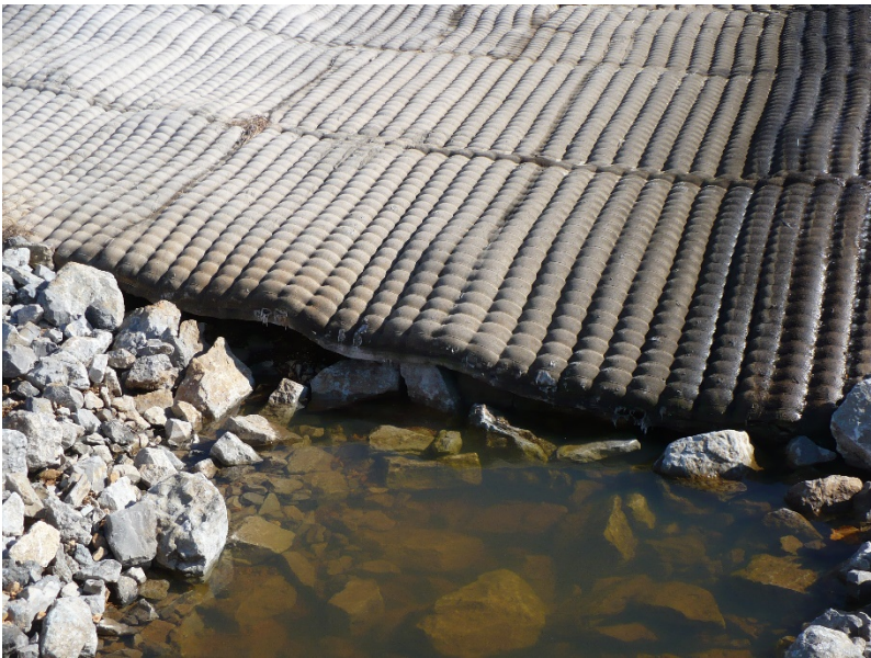
Photo #19 – undermining of SW letdown channel
