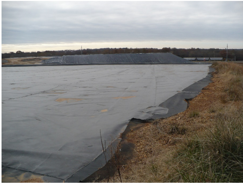
Photo #5 – exposed liner over inactive areas
