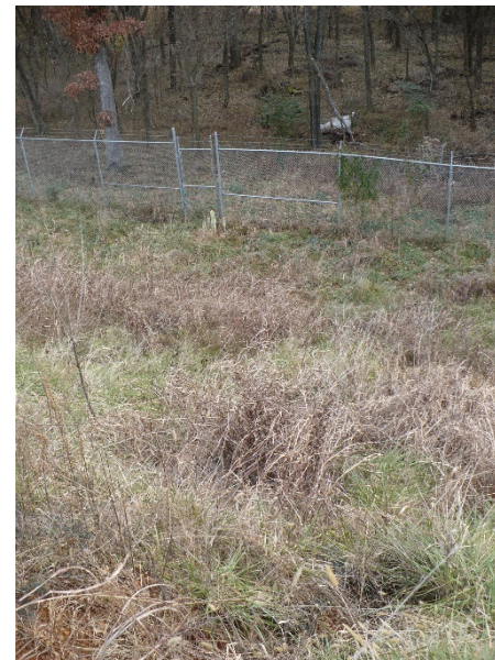
Photo #8 – erosion gully on east containment berm
