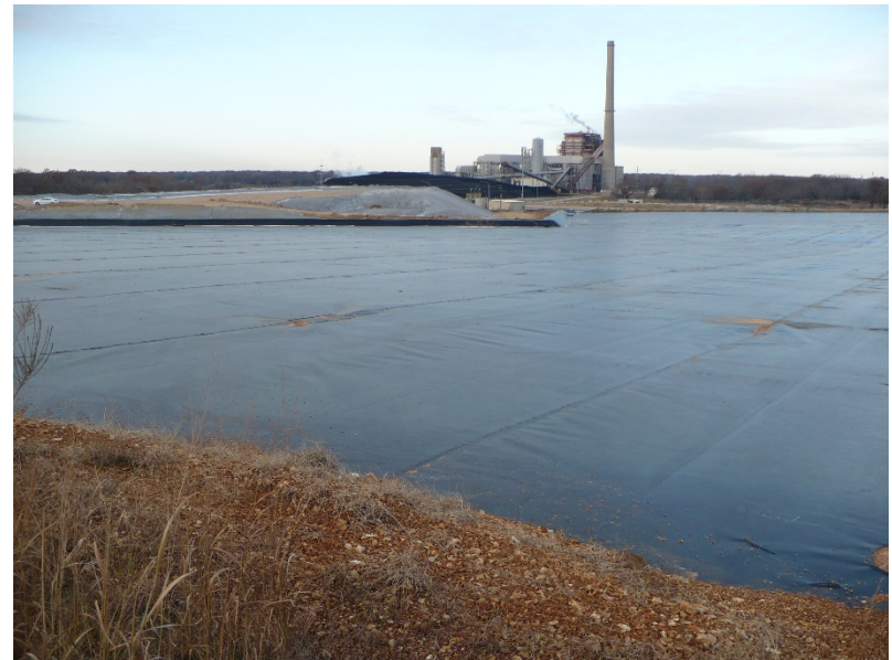
Photo #4 – exposed liner over inactive areas
