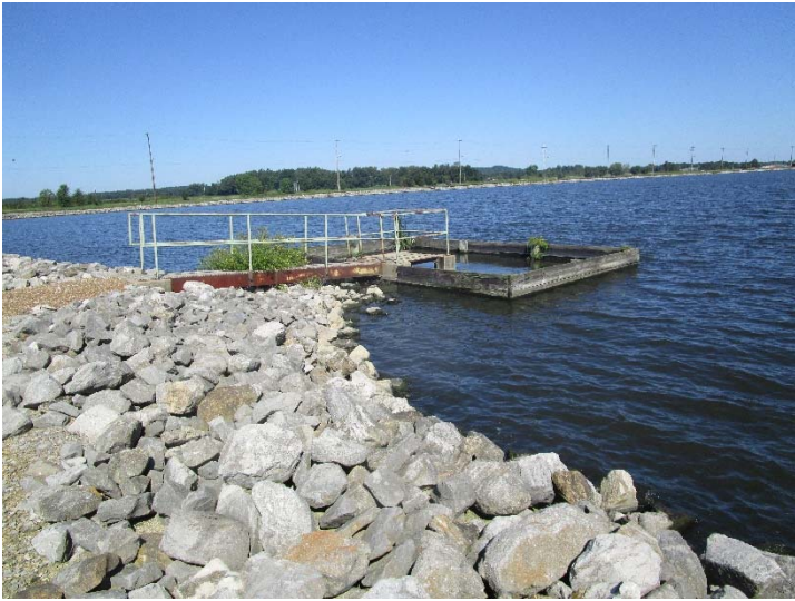
Photo #5W – main discharge structure. p.s. the vegetation shown in the photo was removed during the inspection
