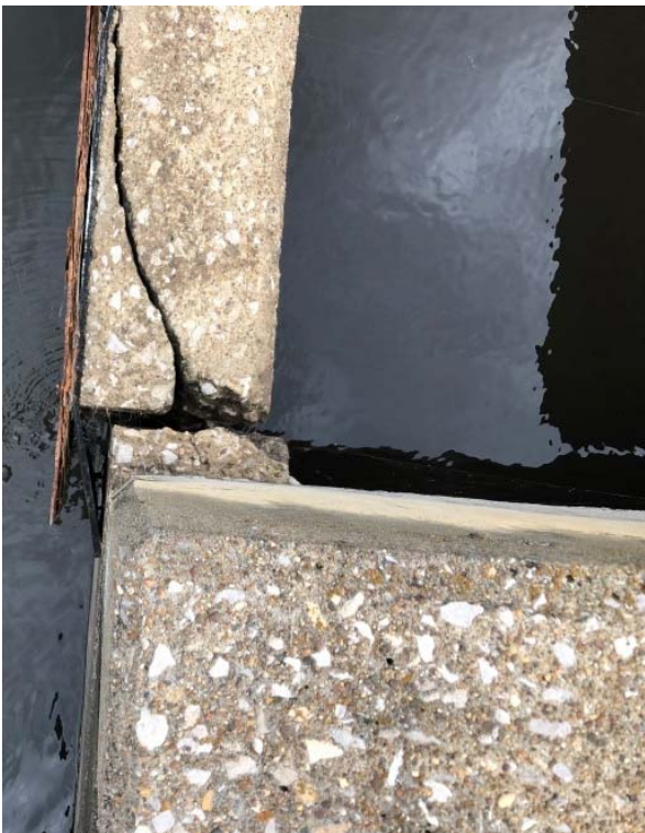
Photo #7WW – old displacement of concrete weir – rebar is still engaged.
