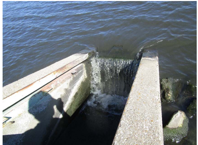
Photo #4W – low level drain operation at full pond
