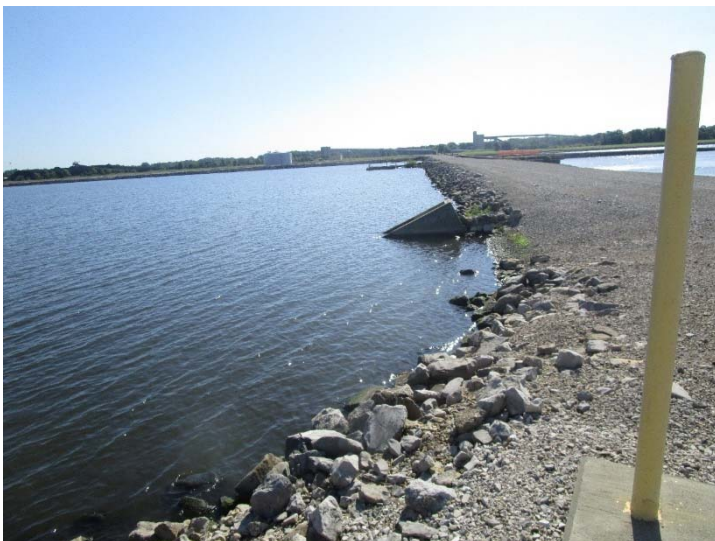
Photo #7W– discharge structures at full pond
