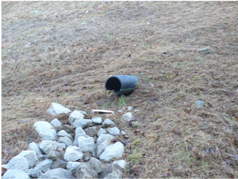
Photo #13 –Outlet pipe from North Sediment pond
