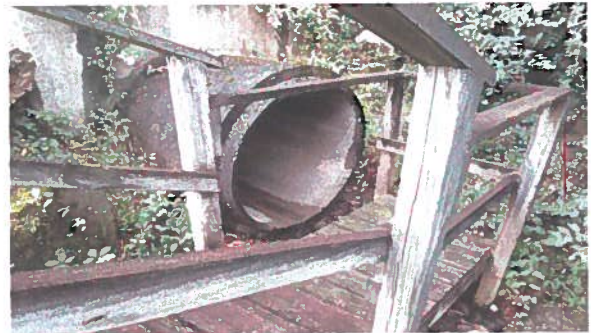
Photo 12- Typical view of the closed primary discharge pipe from the stage one raising. The discharge from the pipe was estimated to be 0.5 gpm and was visually clear.
