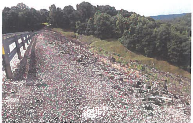
Photo 4 – Typical view showing good conditions of the left groin and stairwell access to piezometers PP10s and PP10d.
