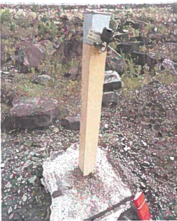
Photo 9-Typical view of piezometer 94-1 showing piezometer-tag number and locked casing protector. The concrete pad is undermined and requires replacement.
