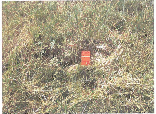
Photo 8– Typical view of along the right groin ditch of the minor slip showing no significant change from previous inspections. Discharge from this area was estimated to be 0.25 gpm and was visually clear.
