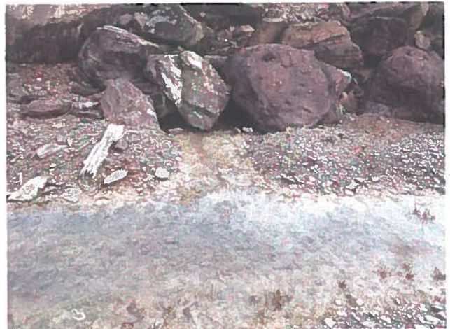
Photo 10- Typical view of the wet weather spring along the toe of the downstream face at the 716 bench.
