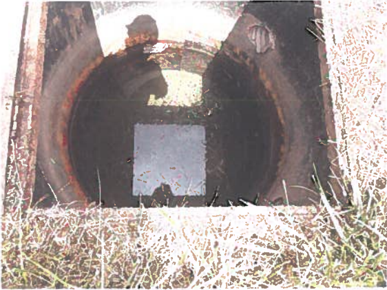
Photo 13- Typical view of the stilling basin that collects seepage from the foundation drainage blanket.
