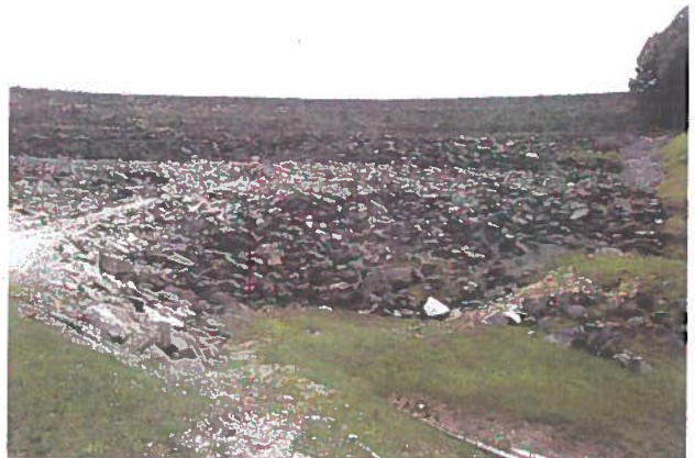
Photo 6 – Typical view showing good conditions of the downstream face showing the oversized rip rap.
