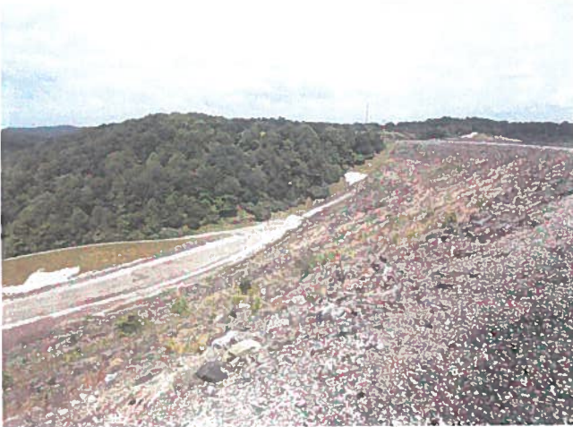
Photo 7 – Typical view showing good conditions of the slip repair in the right groin ditch and a more recent repair along the site access road ramp to the 716 Bench.
