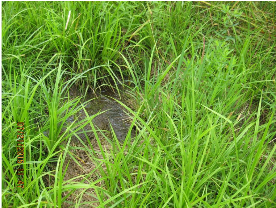
Photo 46: East Wastewater Pond, east dike: water along exterior toe.
