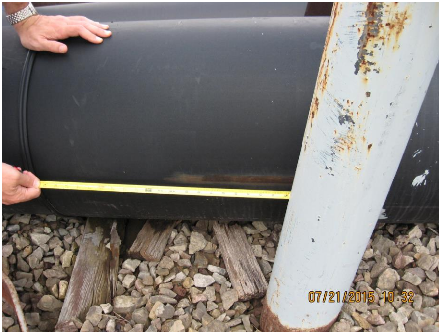
Photo 9: Bottom Ash Ponds: evidence of movement along bottom ash inlet pipes due to thermal expansion.
