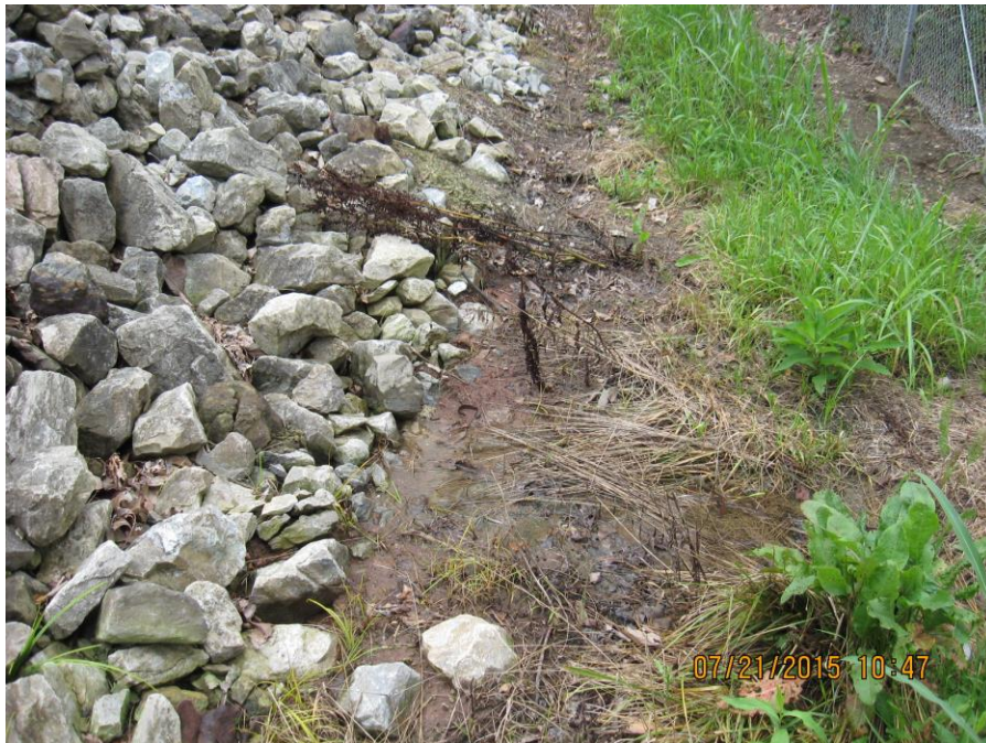
Photo 16: Bottom Ash Ponds, north dike: water near the exterior toe.
