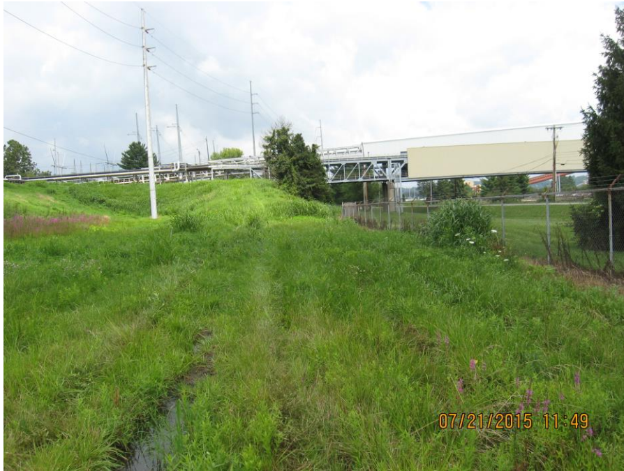
Photo 49: East Bottom Ash Pond, east dike: water along exterior toe.
