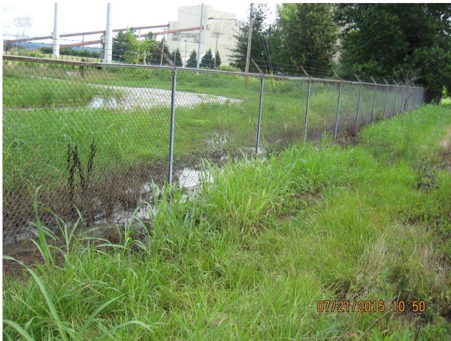
Photo 18: Bottom Ash Ponds, north dike: water near the exterior toe.
