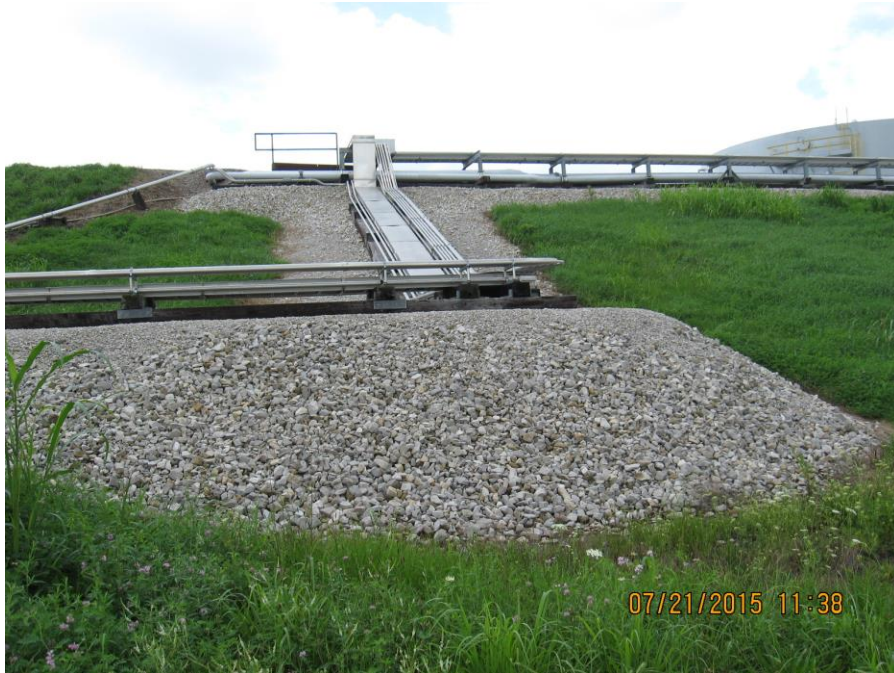
Photo 45: East Wastewater Pond, east dike: piping along exterior slope.
