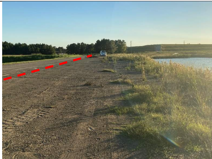
Photograph 2: View along upstream slope, looking right. Superimposed line approximates the original crest upstream shoulder, thus demonstrating the extent of overbuild which has occurred over the original upstream slope.
