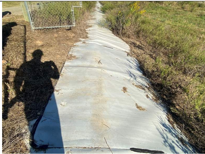
Photograph 14: View of minor abrasion damage of the geosynthetic liner where equipment enter pond through gate at left.
