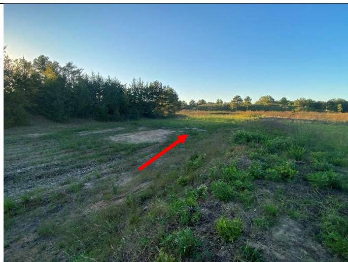
Photograph 9: View of primary emergency spillway, looking upstream. Arrow points to overflow weir location. Note rutting at left side of photo.
