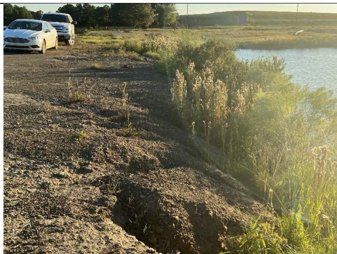
Photograph 3: Close-up view of upstream edge of upstream slope overbuild. Note erosion gullies. Since gullies have formed in the overbuild material, they are not considered problematic.
