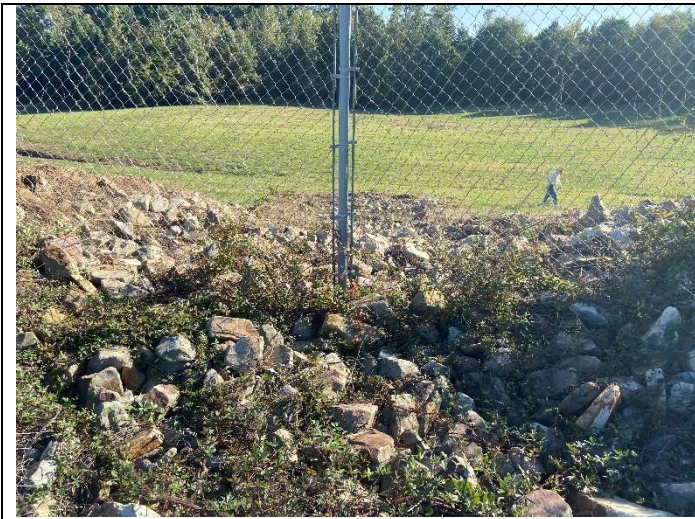
Photograph 10: View of emergency spillway outlet channel, looking downstream. Note crest fence partially blocks the spillway weir.
