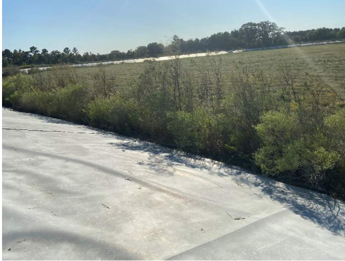
Photograph 5: Example woody vegetation growing at toe of geosynthetic liner toe-in on upstream slope.
