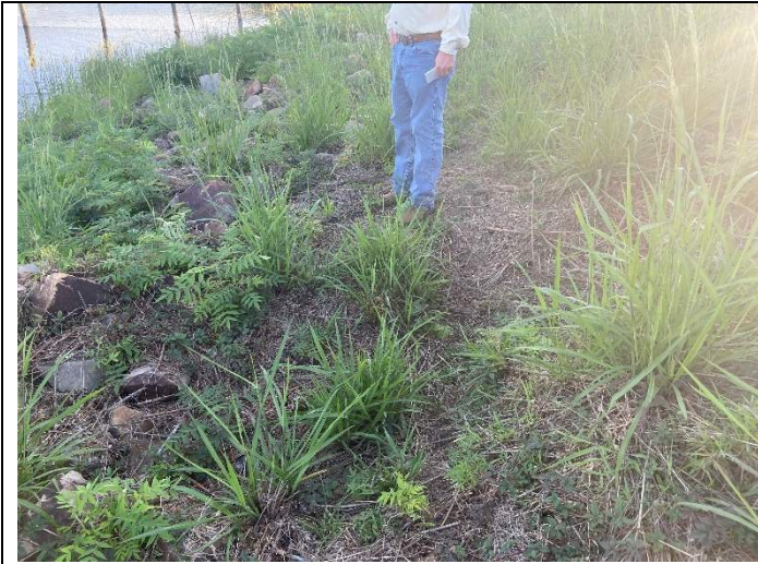
Photograph 7: Example of poor vegetation coverage on downstream slope, near the transition to the rock riprap slope protection. Multiple animal burrows were noted in this area.
