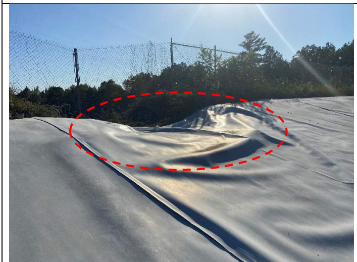
Photograph 9: View of emergency spillway weir. Note bubbling of geosynthetic liner.
