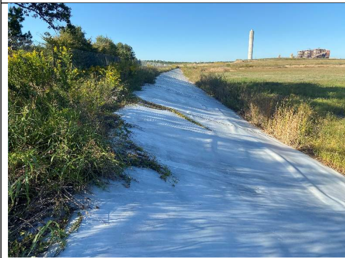
Photograph 11: Typical view of crest and upstream slope on west embankment. Note crest is overgrown with vegetation.
