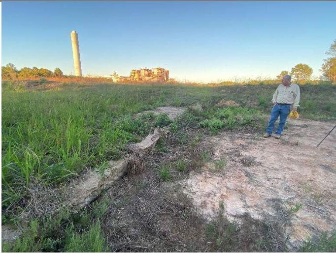
Photograph 11: Close-up view of primary emergency spillway overflow weir. Note undermining damage on upstream and downstream faces, and overall irregularity of the weir.
