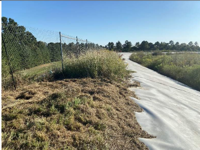
Photograph 6: View of crest where mowing operation had stopped. Beyond this point, the crest of the embankment was overgrown with vegetation and could not be thoroughly inspected. East embankment, near transition to south embankment.
