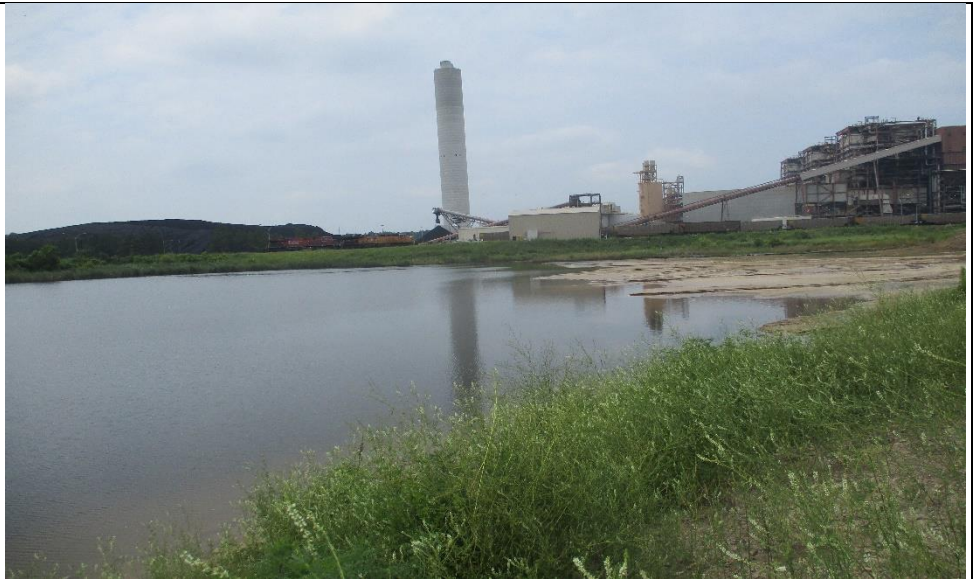
Photograph No. 10 The upstream slope of the north dike supporting the railroad.
