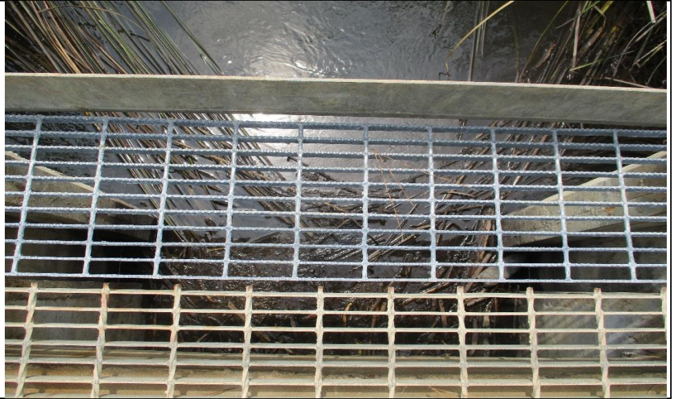
Photograph No. 15 Overflow weir at the discharge structure.
