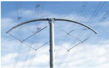
BOLD Transmission Line
