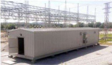
Drop in Control Module
