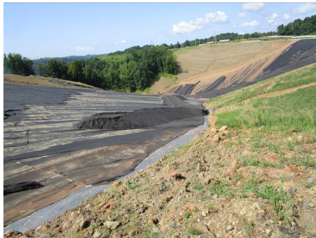
Photograph 5: View of the erosion occurring in the eastern groin of the clay berm area and the limits of the new construction.
