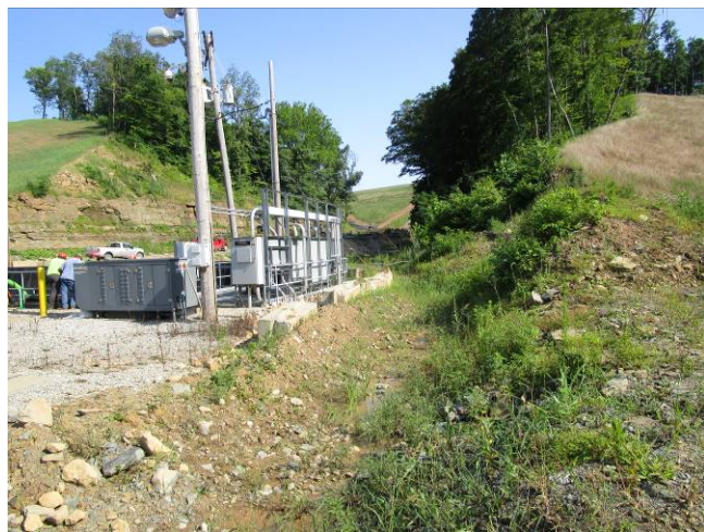
Photograph 9: View of the open channel spillway between the south pond forebay and the south pond.
