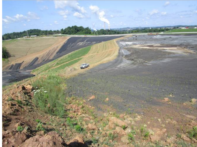
Photograph 4: Overview of the clay berm, facing west. The bare soils define the recently placed clay material.
