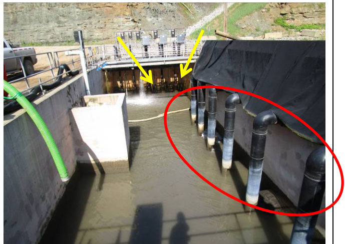
Photograph 8: View of the leachate collection sump. The leachate collection pipes are circled in red, and the leachate pumps are indicated by the yellow arrows.
