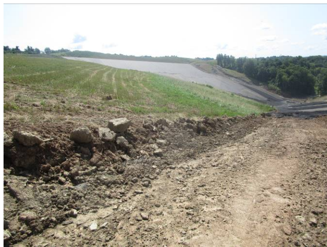
Photograph 6: View of the erosion rill on the dirt access road on the clay berm.
