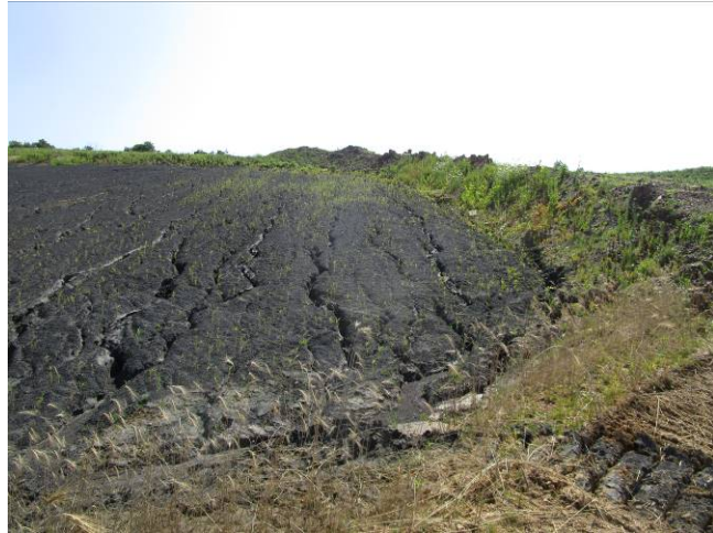
Photograph 1: View of the erosion rills on the protective cover material on the north and east face of the Phase 2 area.
