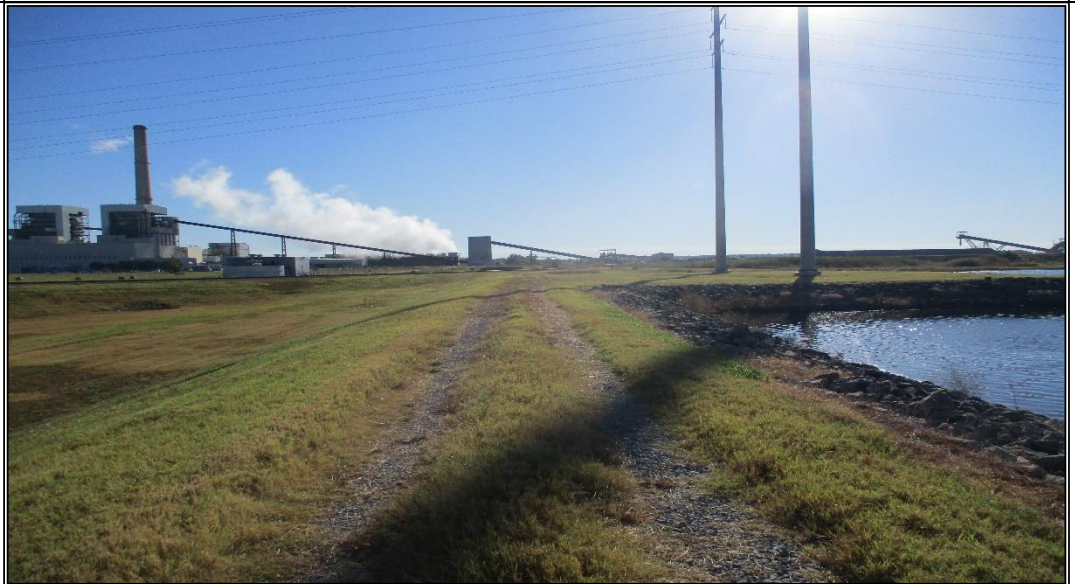
Photograph No. 5 Typical condition of the crest of the northwest dike section (looking east).
