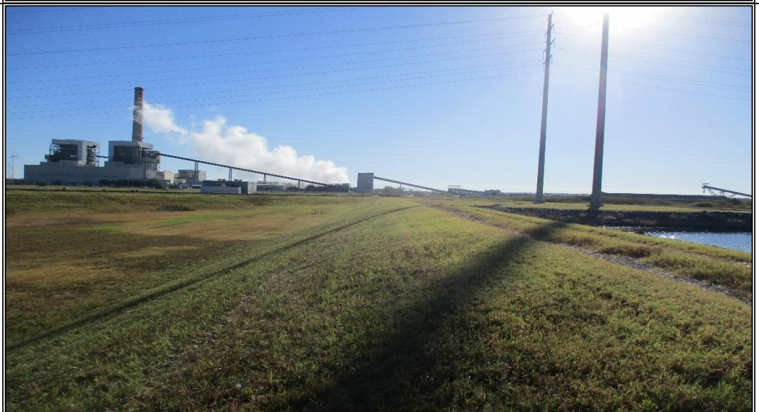
Photograph No. 6 Typical condition of the downstream slope of the northwest dike.
