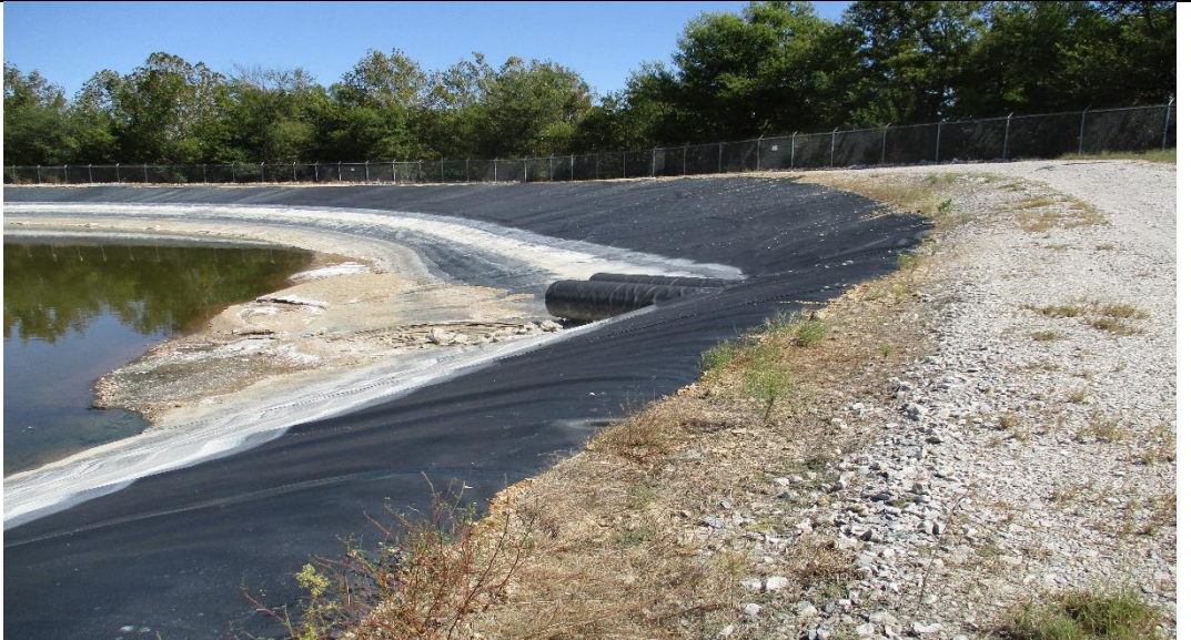
Photograph No. 22 Interior slope and south runoff water pipe at Basin C.
