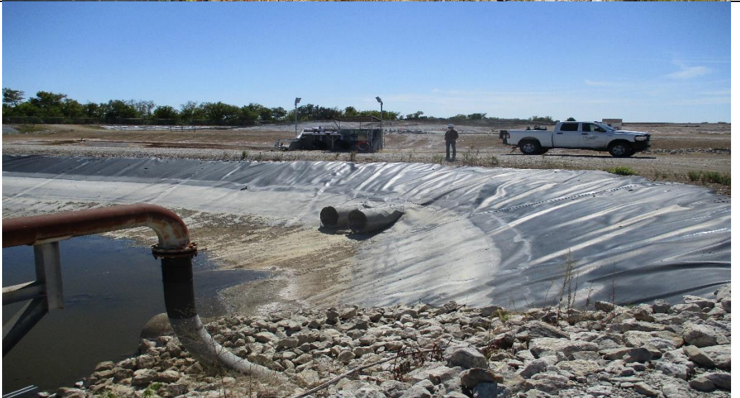
Photograph No. 23 Interior slope and north runoff water pipe at Basin C
