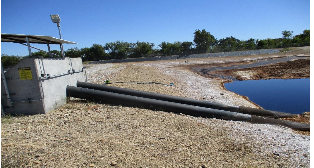
Photograph No. 17 The leachate pump system.
