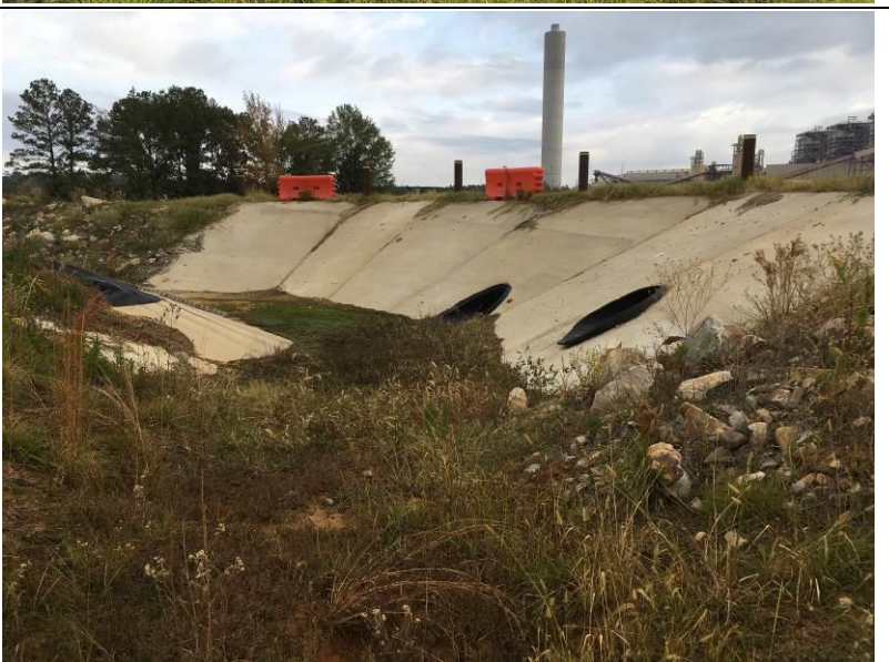
Photo # 8 View of the 30- and 36-inch Storm Water Pipes Located in Northeast Corner of Landfill Perimeter Ditch. Notice Sediment Buildup in Ditch and In Front of Pipe Inlets.
