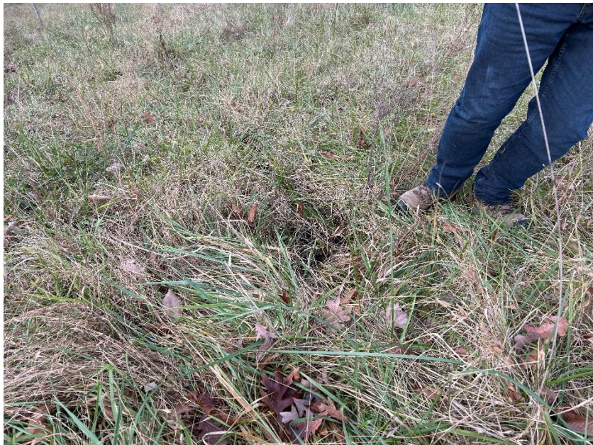
Photo #7–Sequence 4 North Valley Embankment Slope/Erosion
