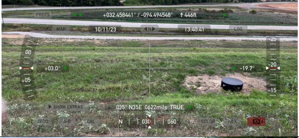
Photograph No. 32 Landfill Cover – view of one of the let-down catch basins inlets on top of 1999 area.
