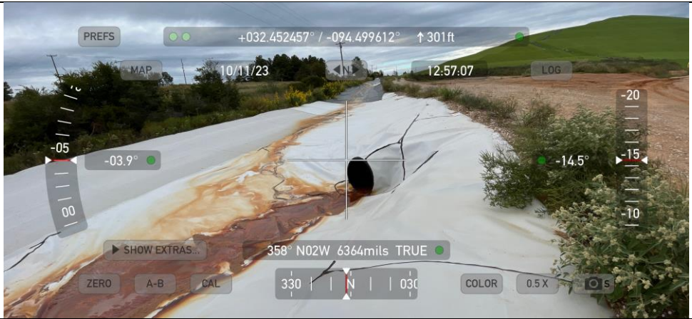
Photograph No. 26 View of the non-contact water perimeter ditch on the west side of landfill. Note iron stain in geosynthetic.
