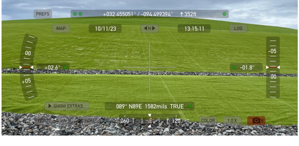
Photograph No. 29 View of cell 2015 showing final cap and cover. (looking northeast)
