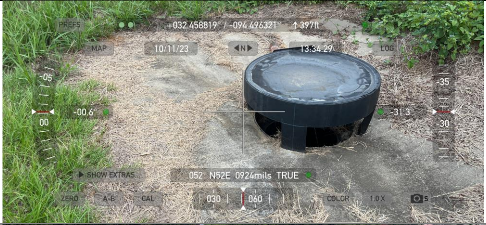
Photograph No. 31 View of one of the let-down catch basins inlets on top of 2005 area.
