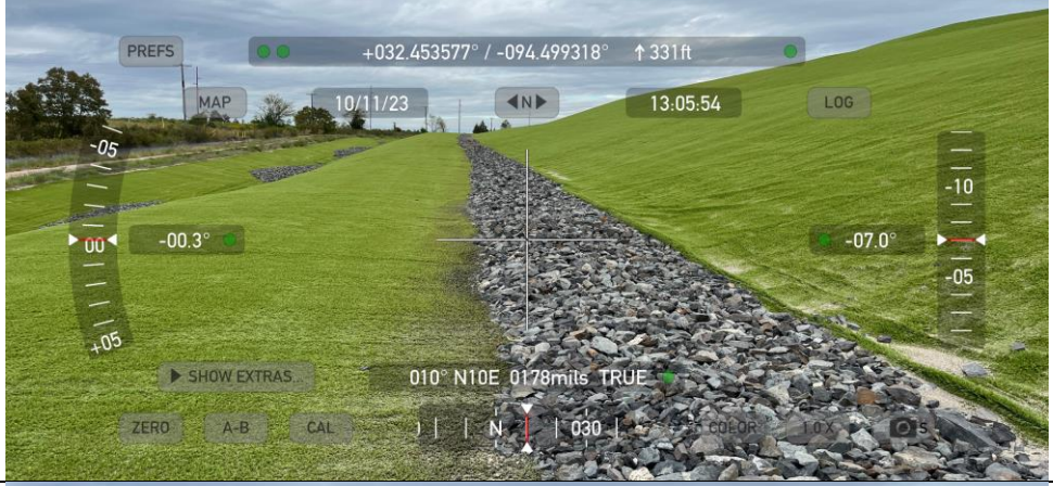
Photograph No. 28 View of cell 2015 showing final cap and cover with a rock lined bench on the closure turf material. (looking northeast)
