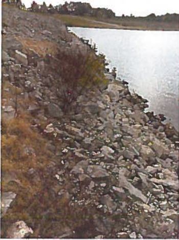
Photo 7 – several dead woody vegetation to be removed on downstream slope.
